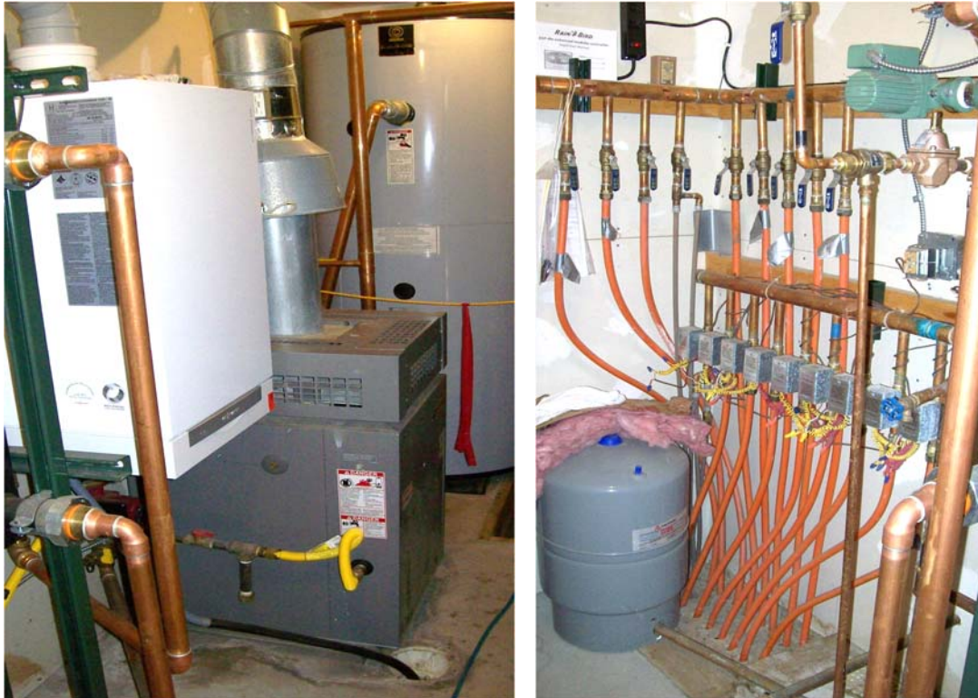
Central boiler for heat and another for hot water, together with a hot water storage tank.
